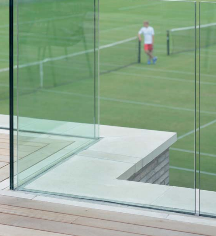
External terrace glass balustrading detail with precast concrete parapet coping by Specialist Precast Products.
