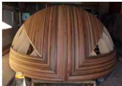
Figure 1.6 (top) Douglas fir stringers are fixed into notches cut in the frames
